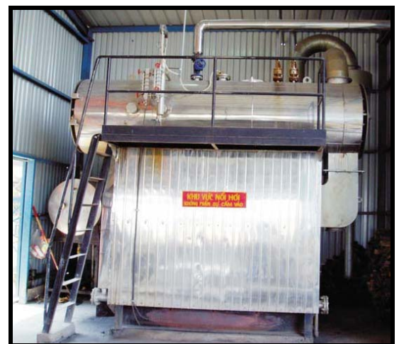
M.E.S. PLANTS Site: GOLDEN MANUFACTURERS BOILA CIRCLE, KALABO INDUSTRIAL ESTATE NASINU, FIJI 1x 4MW Wood Waste Steam Boilers Complete Packaged Steam Plant
